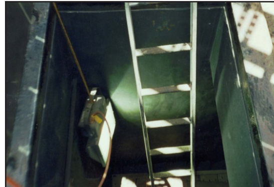
ARC specified by plant engineer
